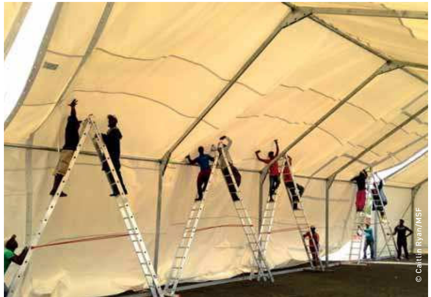
Monrovia, Liberia. Construction teams building what would become ELWA 3, the world’s largest Ebola management centre with 250 beds.
